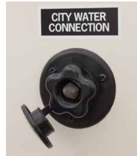
Typical city water fill
