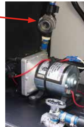
Typical water pump installation
